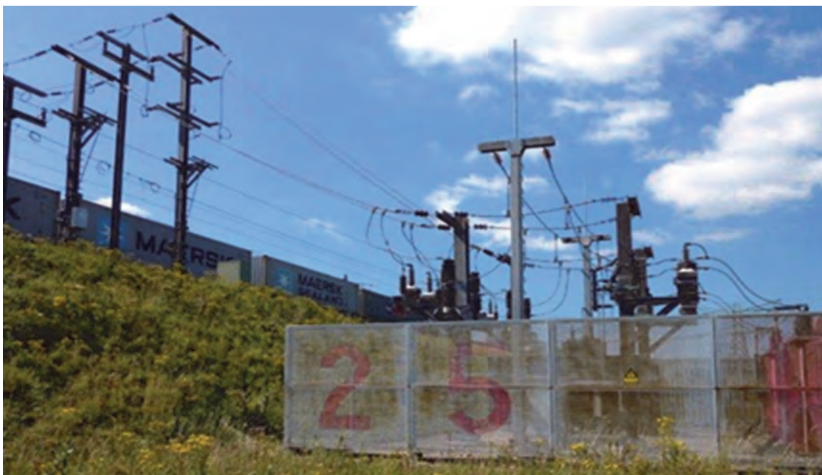
25 kilo Volt power supply station at harbour line Rotterdam Source: Keyrail
