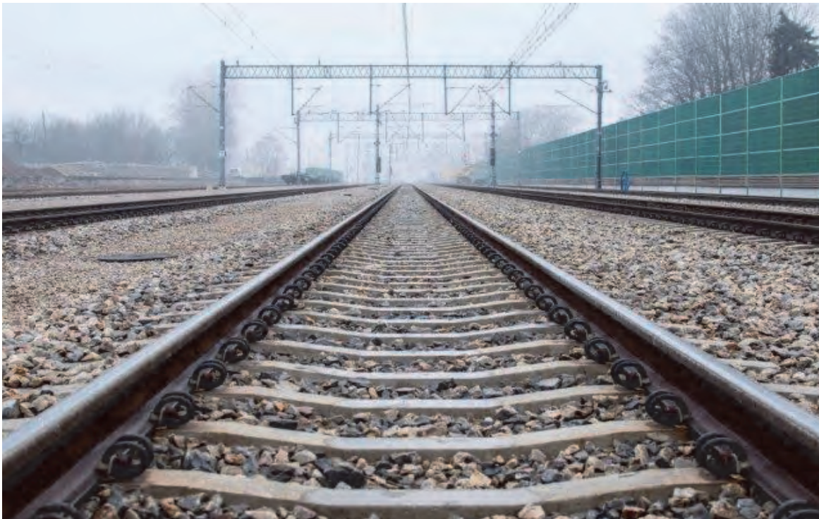
Jaktorów – Żyrardów on the railway line between Warsaw and Łódź Source & Copyright: PKP Polskie Linie Kolejowe S.A.
